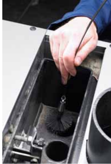
Clean the boiler convector by brushing the convector pipes clean.
